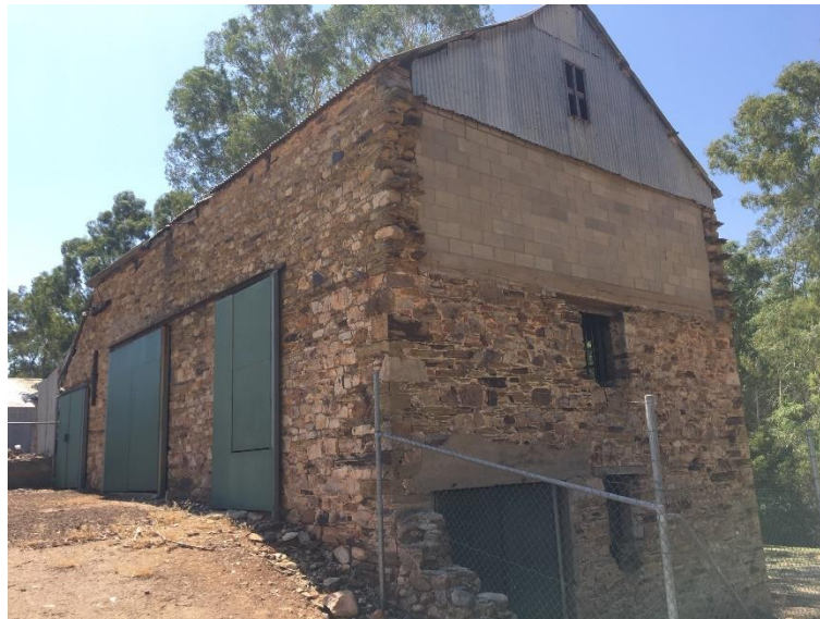
North-western and south-western elevations of the mill. Note the corrugated iron sheeting to gable end and concrete block infill wall.
