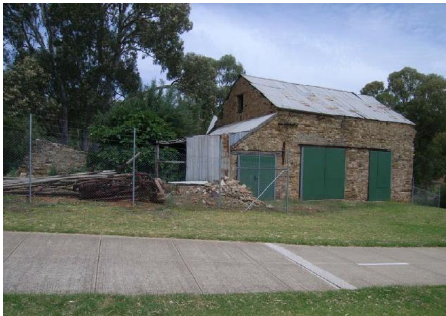
North-western elevation of the mill. The green steel doors were installed to secure the site.
