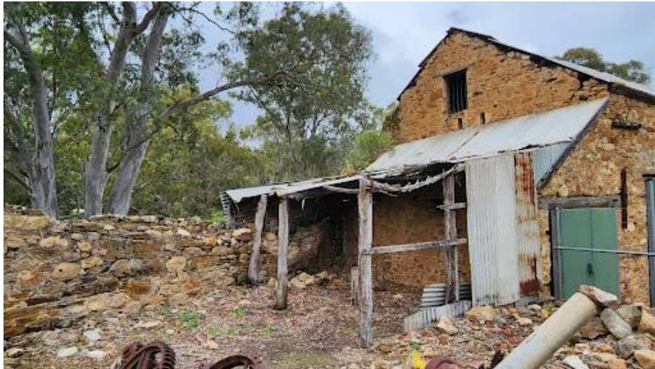
Timber-framed lean-to addition to the north-eastern elevation. The steam boiler was likely positioned in this area.
