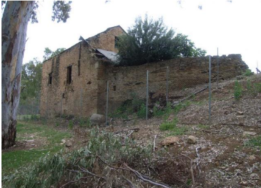
South-eastern elevation with remains of the curved stone flue wall on the right.
